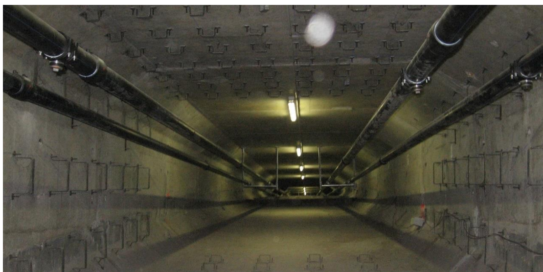
Figure 9. General view of the external prestressing cables installed in the bridge deck.
