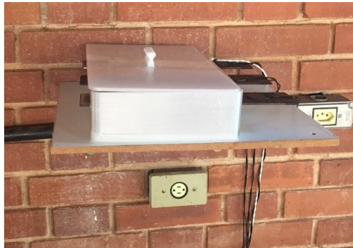
a: Beams inside the control box.
