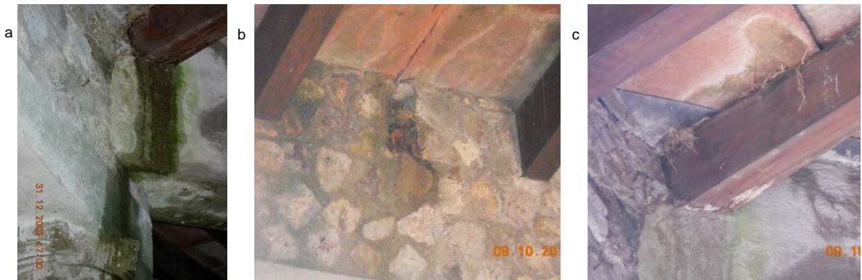
Figure 8. (a) Rafter end support before collapse; (b) End support after collapse; (c) Actual end support conditions of the remaining rafters
