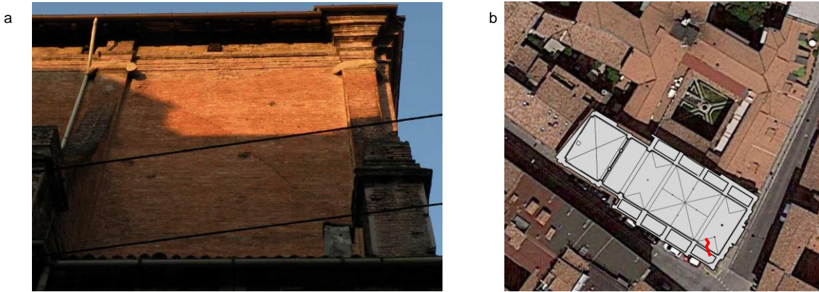
Figure 2. (a) Diagonal crack in the masonry wall at the second level; (b) Position of the Church and its surroundings.
