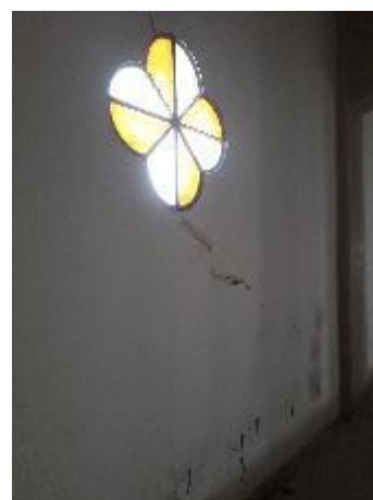
Figure 5: Cracks in side wall
