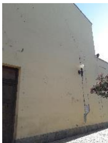
Figure 4: Cracks in the front facade
