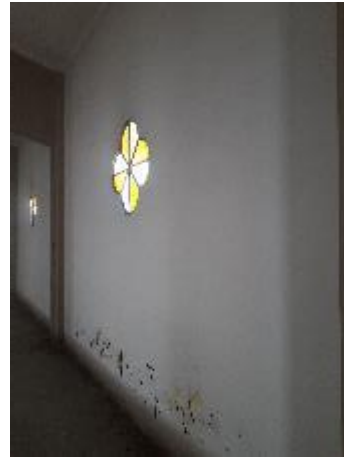
Figura 7: Moisture in walls
