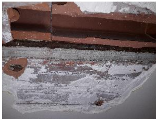
Figure 11: Slab reinforcement corrosion
