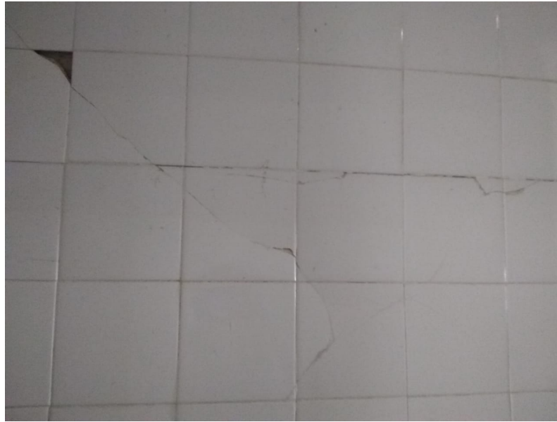
Figure 2. Cracks in ceramic tiles caused by settlement.
