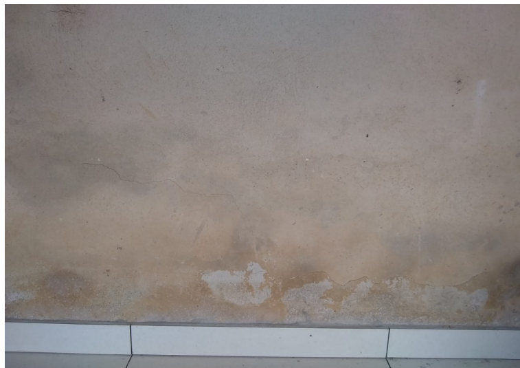
Figure 9. Moisture due to rising dampness from the ground.
