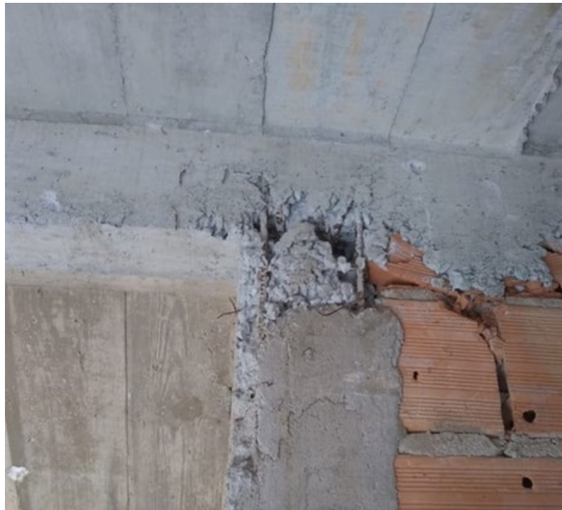
Figure 4. Drill in the beam-column connection that favors the corrosion of the reinforcement.
