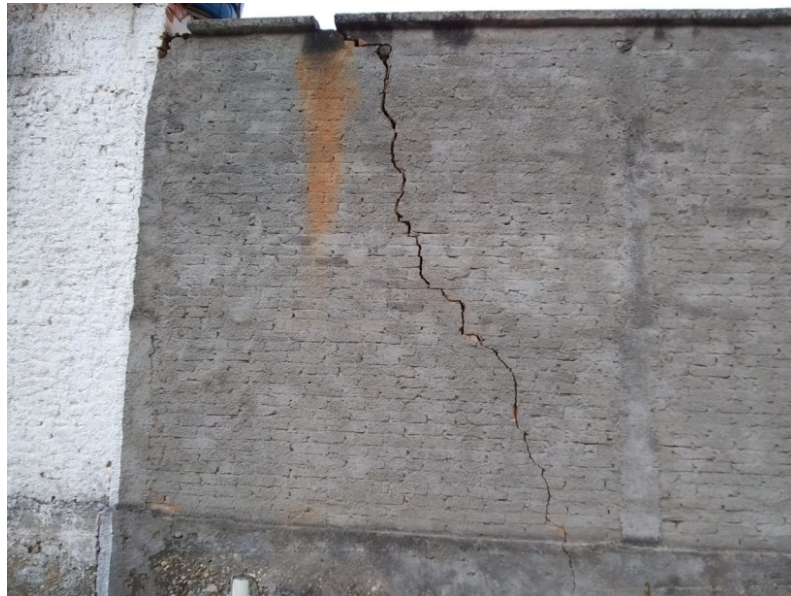
Figure 1. Crack in wall caused by settlement.
