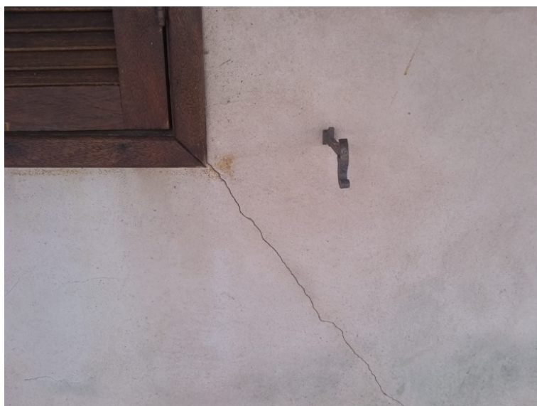
Figure 7. Crack in counter lintels.
