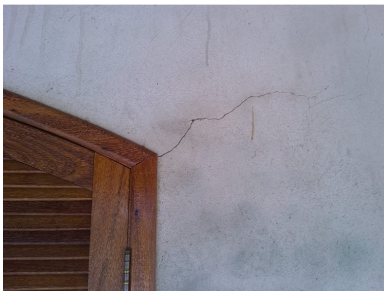
Figure 6. Crack in lintels.
