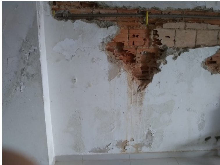
Figure 8. Moisture due to leakage in a water tank.
