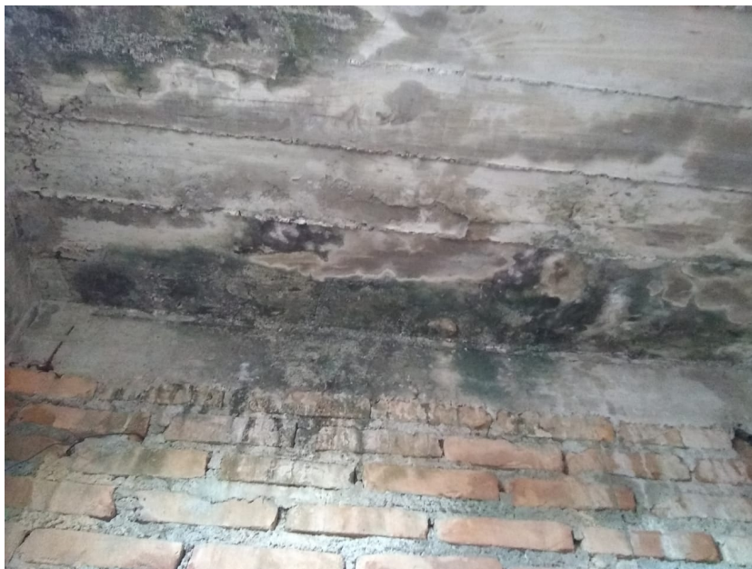
Figure 3. Reinforced concrete slab with mold and stains.
