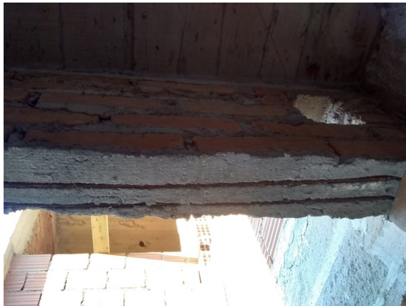
Figure 5. Exposed reinforcement in the frame support beam.
