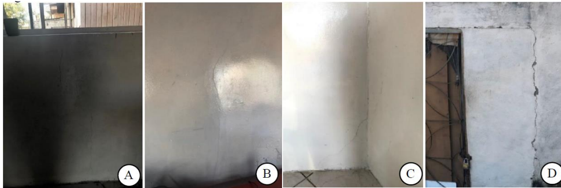
Figure 12 – Cracks found in residence 4.
