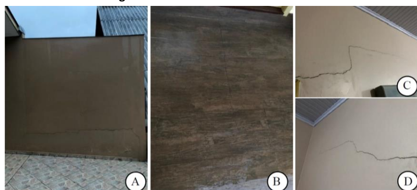
Figure 6 – Cracks found in residence 1.
