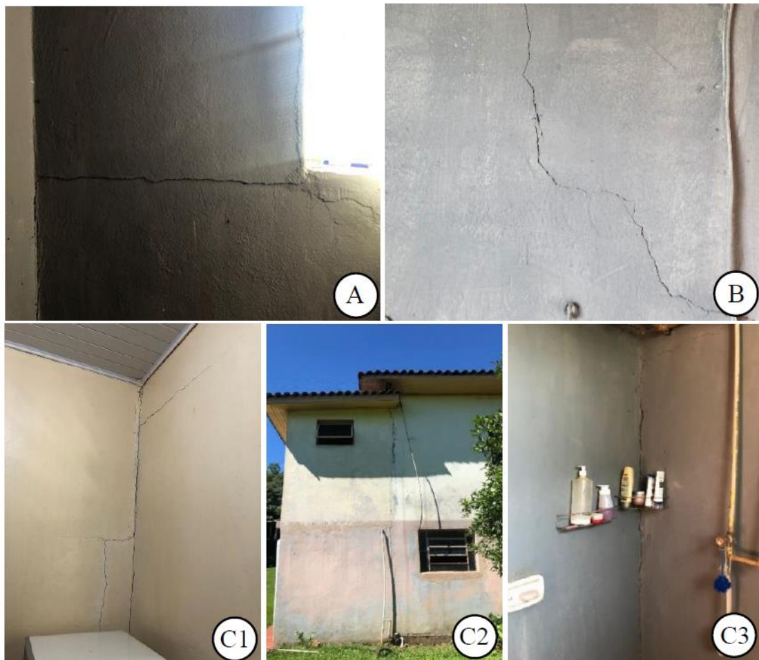
Figure 10 – Cracks found in residence 3.
