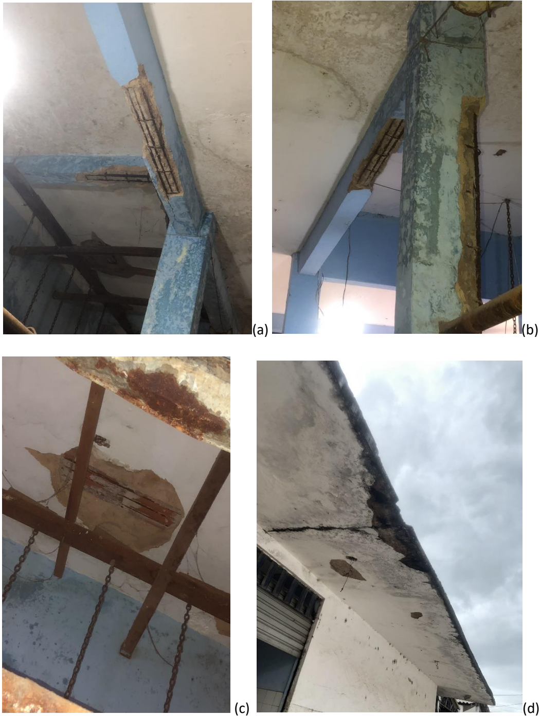
Figure 10 – Corrosion of the reinforcement of the structural elements of the public market.
