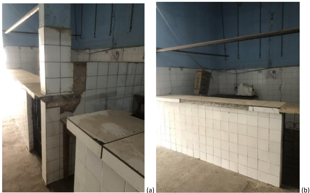
Figure 9 – Detachment of complete parts, in addition to part of the ceramic plates.
