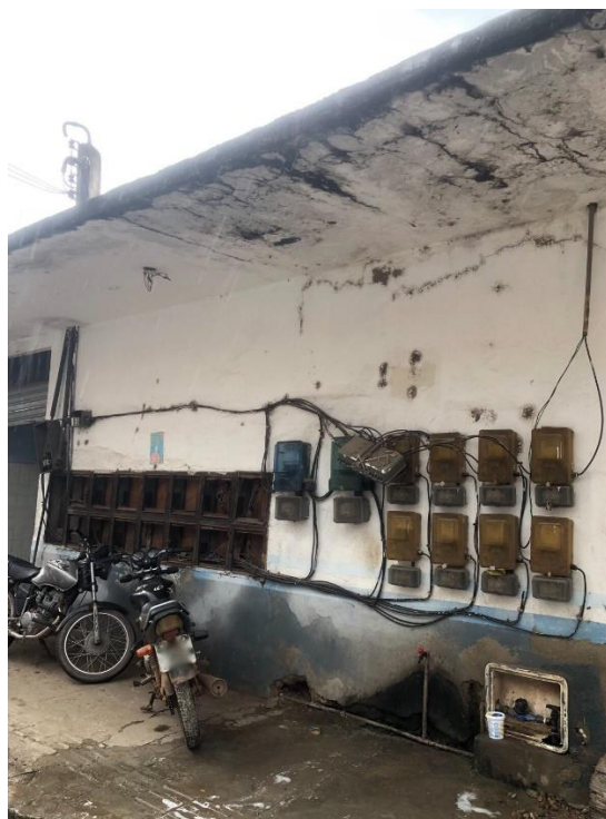
Figure 11 - Corrosion of reinforcement of structural elements of the public market
