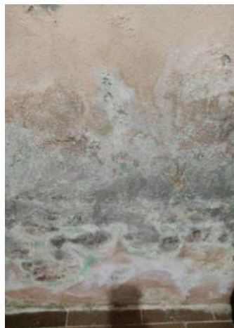
Figure 3 – Efflorescence on a wall.
