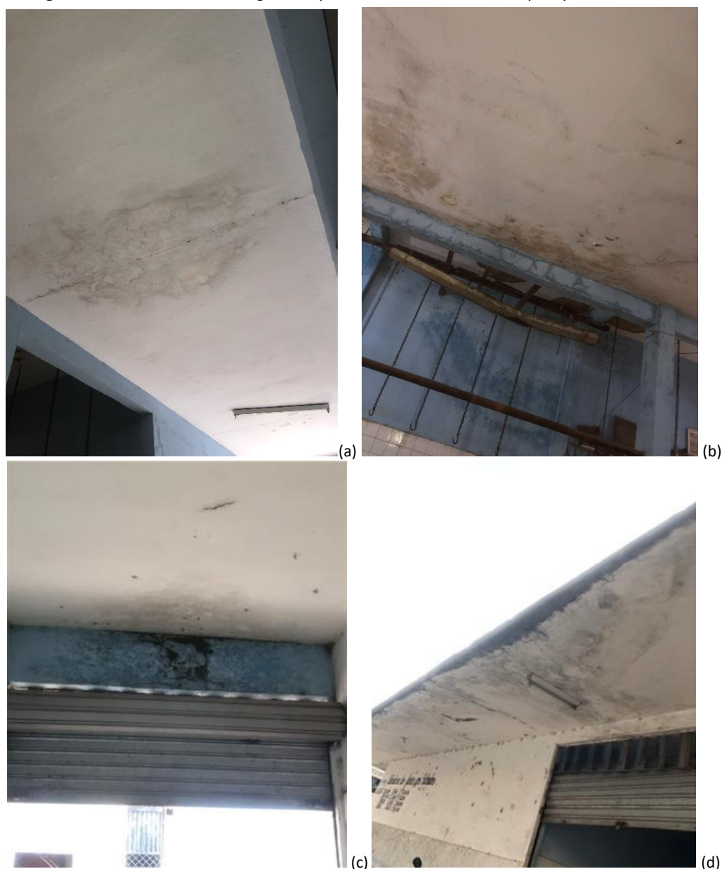
Figure 8 – Stains on the ceiling of the public market in the municipality of Frecheirinha.
