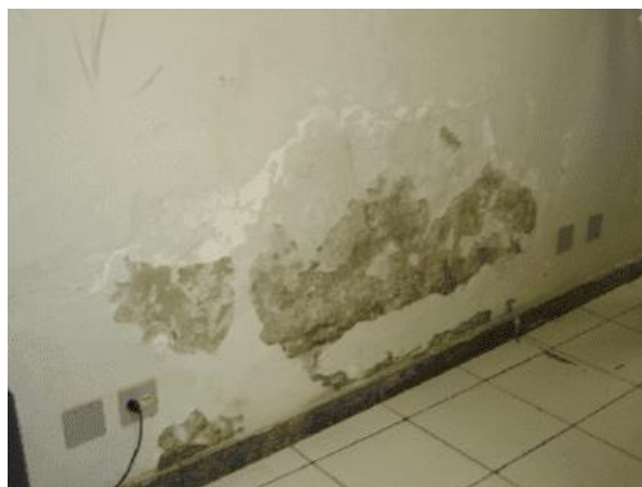
Figure 2 - Presence of stains on a wall.
