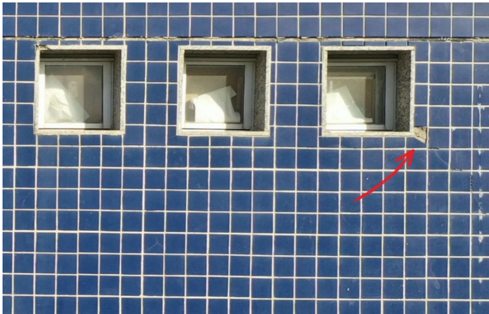
Figure 6 – Cracks in the windows
