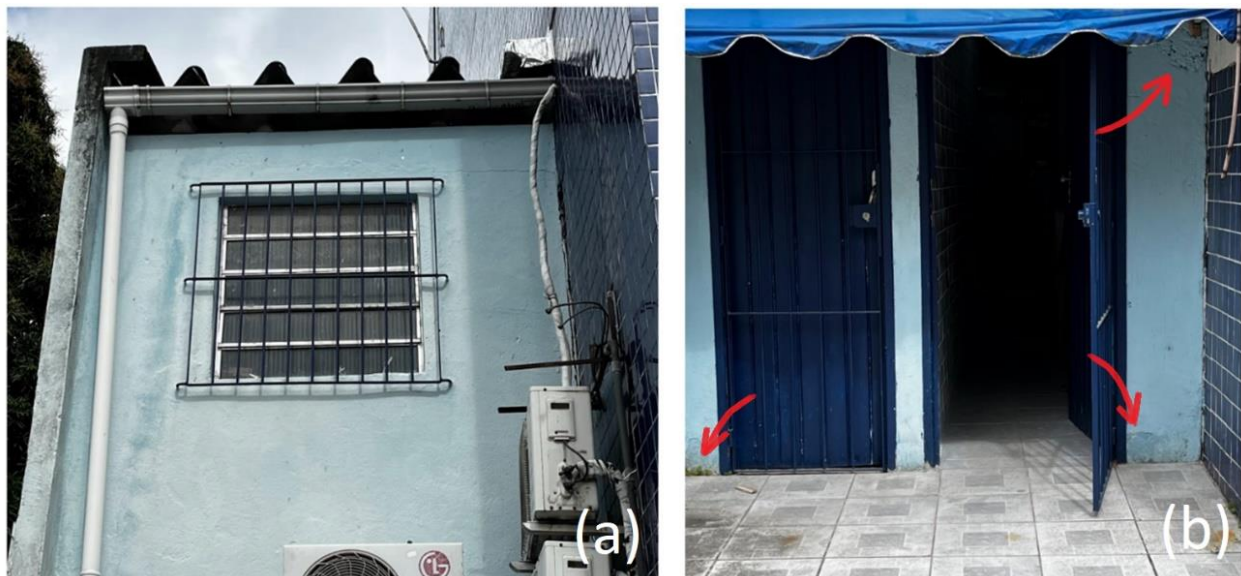
Figure 10 – Grime and moisture stains (a); separation of concrete and vegetation (b)
