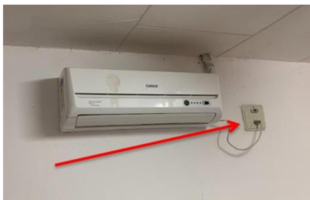
Figure 10 - Educandário air conditioning
