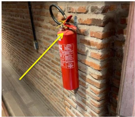
Figure 7 - Extinguisher present inside the Theater
