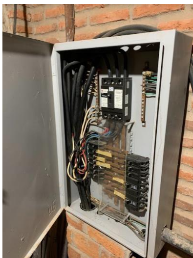
Figure 9 - Electric Theater Board
