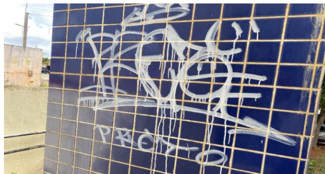
Figure 9 - Visual aspects of the presence of vandalism
