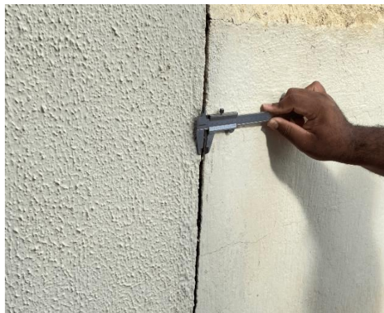
Figure 10 - Longitudinal crack located at the junction of materials
