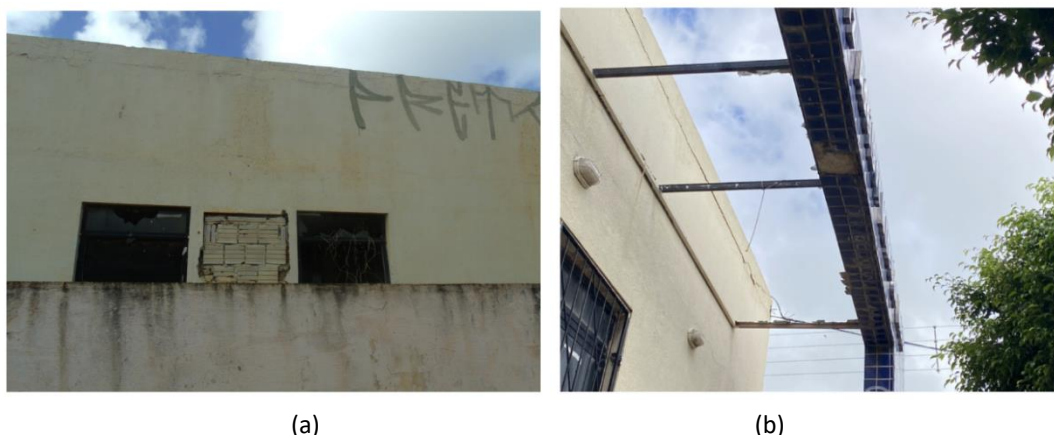
Figure 6 - Visual aspects of pathological manifestations - (a) absence of material and (b) visual pollution/elements not belonging to the original project
