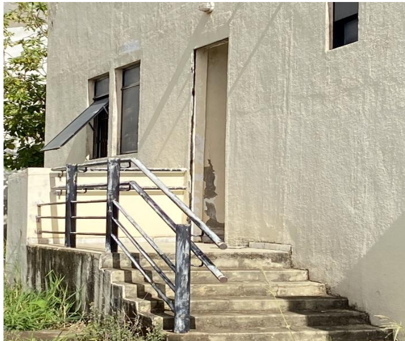
Figure 5 - Visual aspects of the presence of peeling of the pictorial layer
