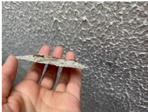
Figure 17 – Insufficient concrete cover
