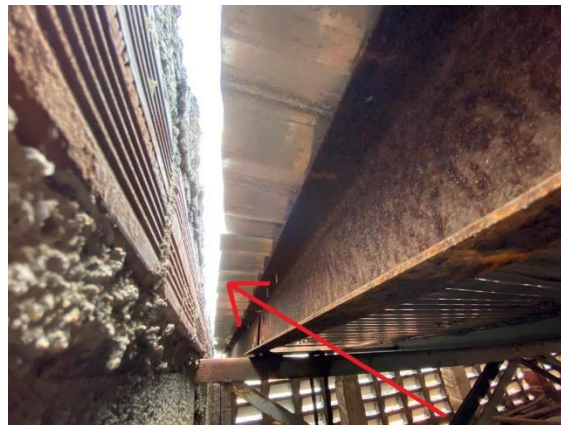
Figure 10 – No elements to prevent rain splashes
