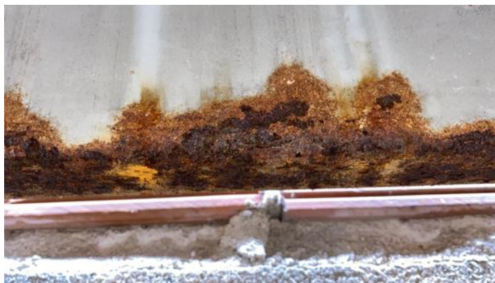
Figure 5 – State of corrosion of the steel section
