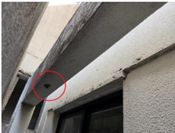
Figure 14 – Beam corrosion area
