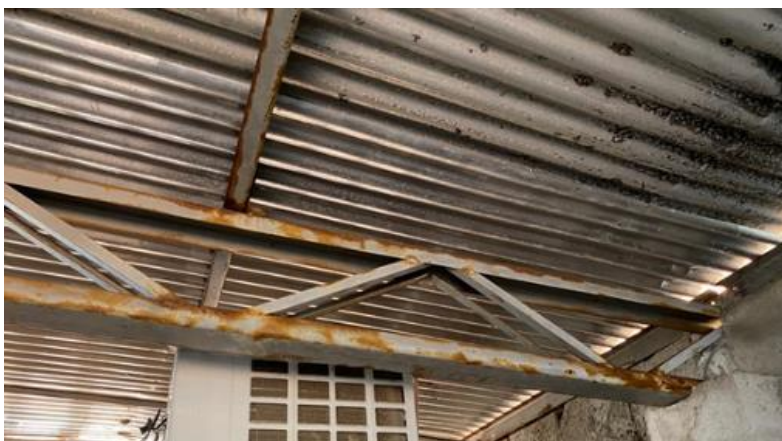
Figure 4 – Corrosion in the steel structure
