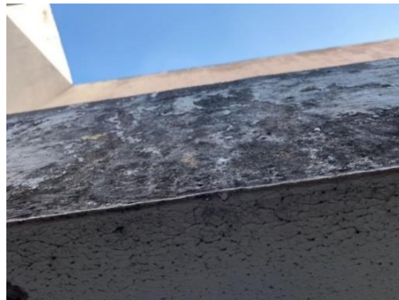
Figure 16 – Absence of drainage elements
