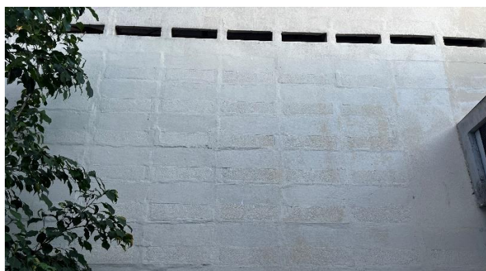
Figure 17 – Marks on the façade
