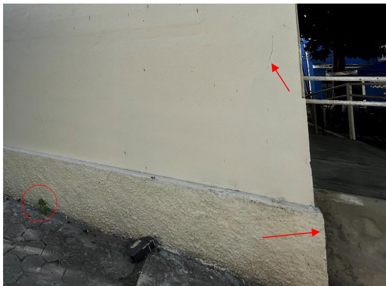
Figure 21 – Building defects of left side façade
