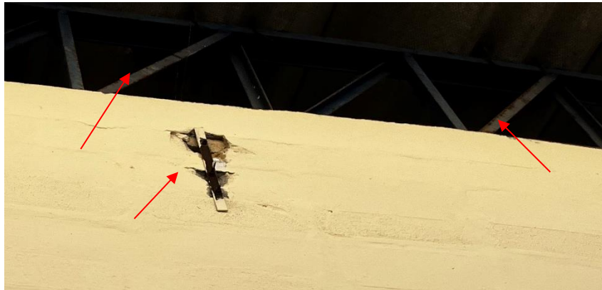
Figure 25 – Pieces with corrosion
