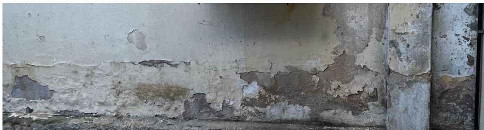
Figure 16 – Fissures and paint detachment
