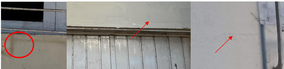
Figure 10 – Fissures on doors and windows
