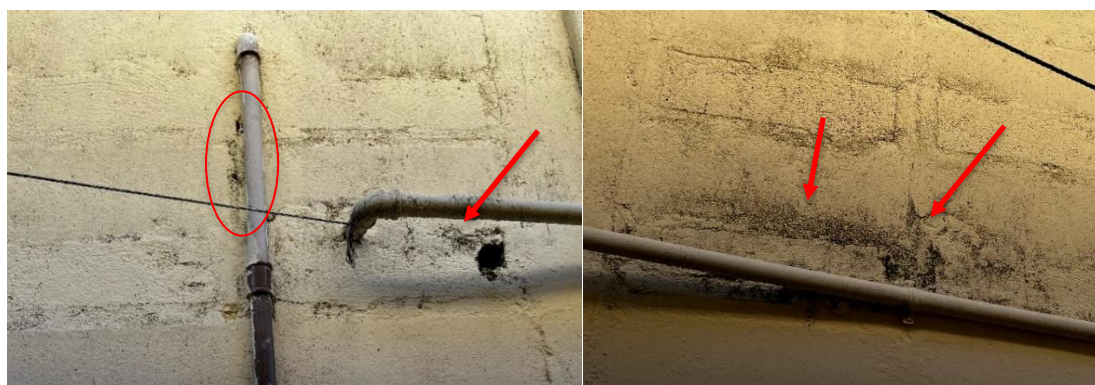
Figure 23 – Dirt and mildew stains
