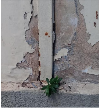
Figure 8 – Corrosion and vegetation
