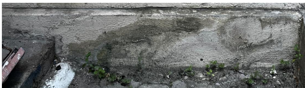
Figure 11 – Dirt and vegetation
