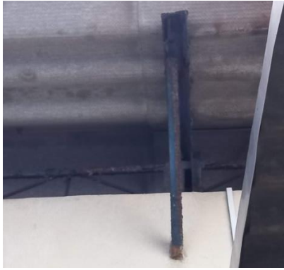
Figure 14 – Pieces with corrosion
