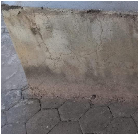
Figure 5 – Fissures on ramp
