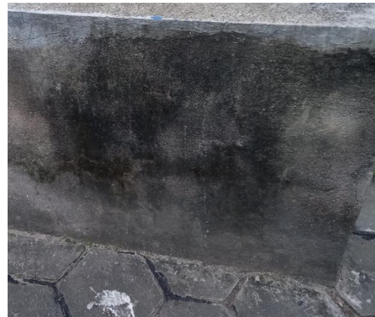
Figure 6 – Dirt on the ramp
