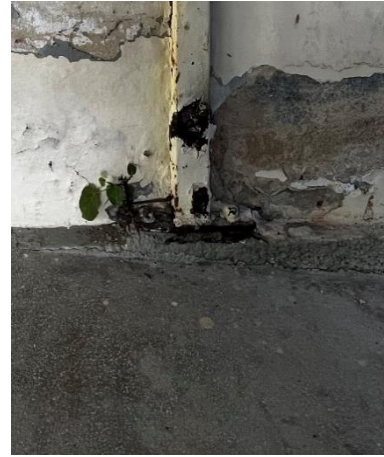
Figure 9 - Corrosion and vegetation on the column
