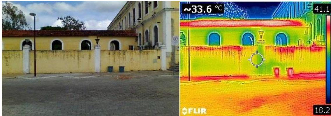
Figure 23 - Thermographic analysis of the wall on the façade of Vale do Acaraú State University (UVA) – Betânia Campus
