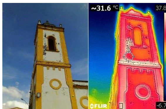
Figure 7 - Verification of manifestations on the lateral facade of the Church of Sorrows.
