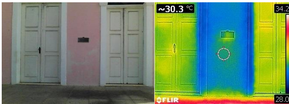
Figure 4 - Verification of possible pathology on the facade of São João Theater.
