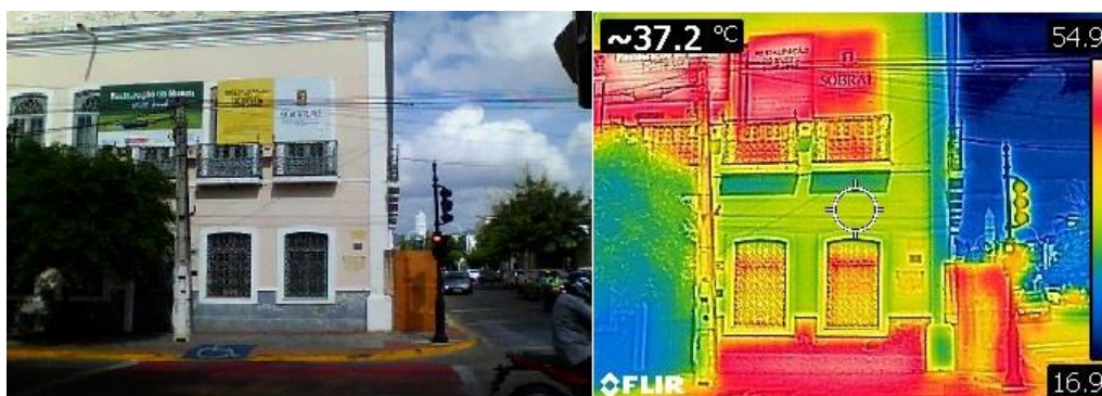
Figure 16 - Verification of pathological manifestations on the facade of the Dom José Museum.
