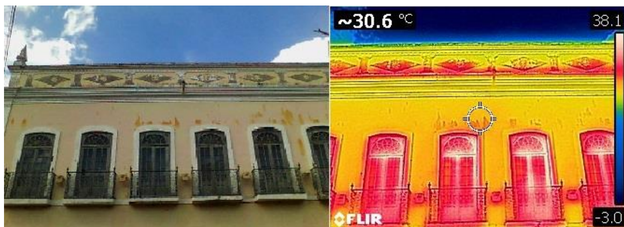
Figure 17 - Verification of pathological manifestations on the facade of the Dom José Museum.
