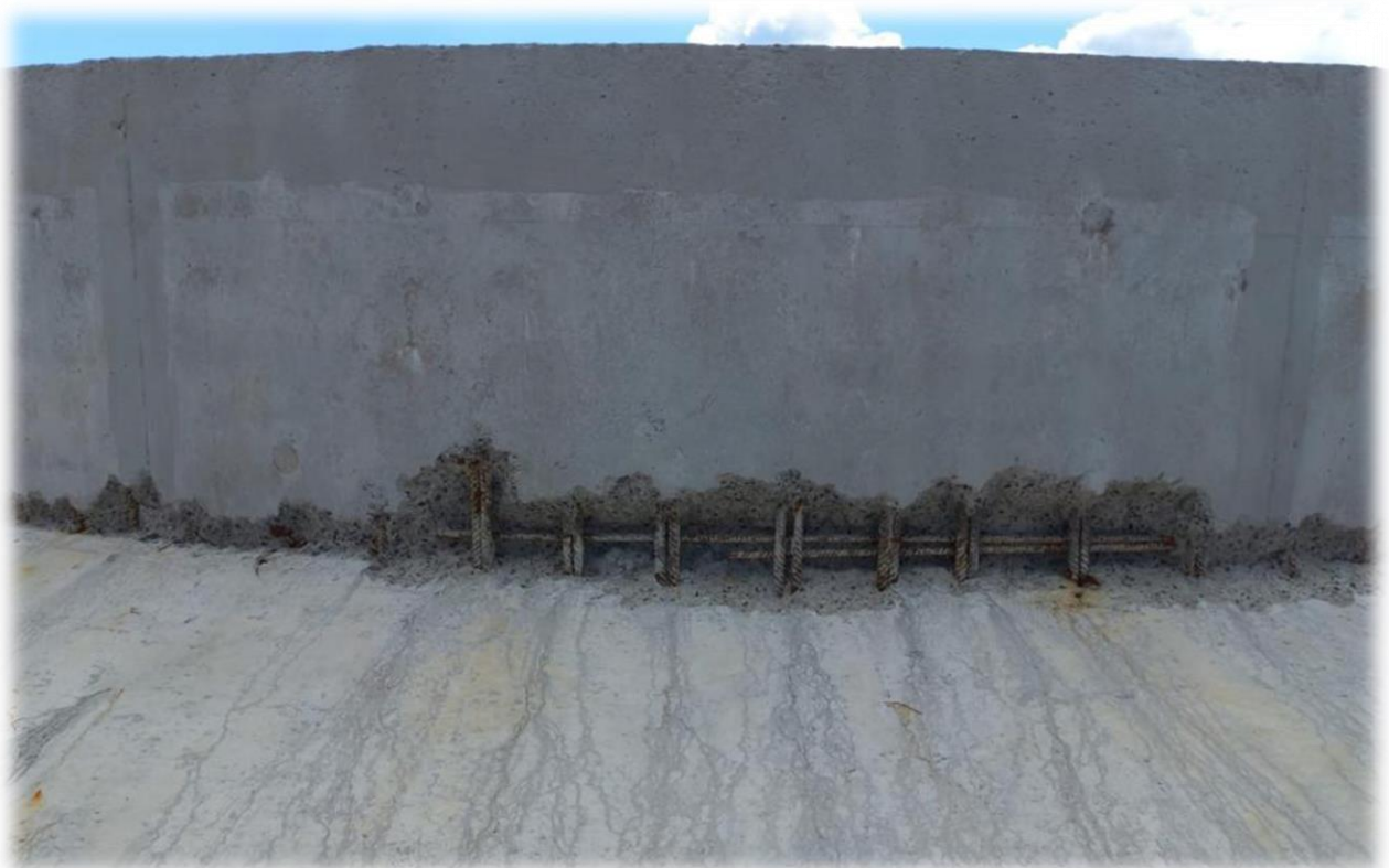
Figure 5 – Example of honeycomb in a wind turbine foundation.
