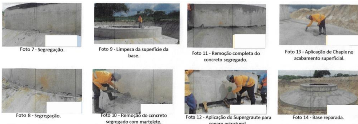
Figure 8 – Repair action reported inspection form.
