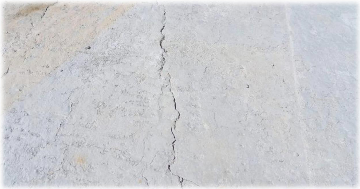
Figure 4 – Example of a crack at the base of a wind turbine foundation.
