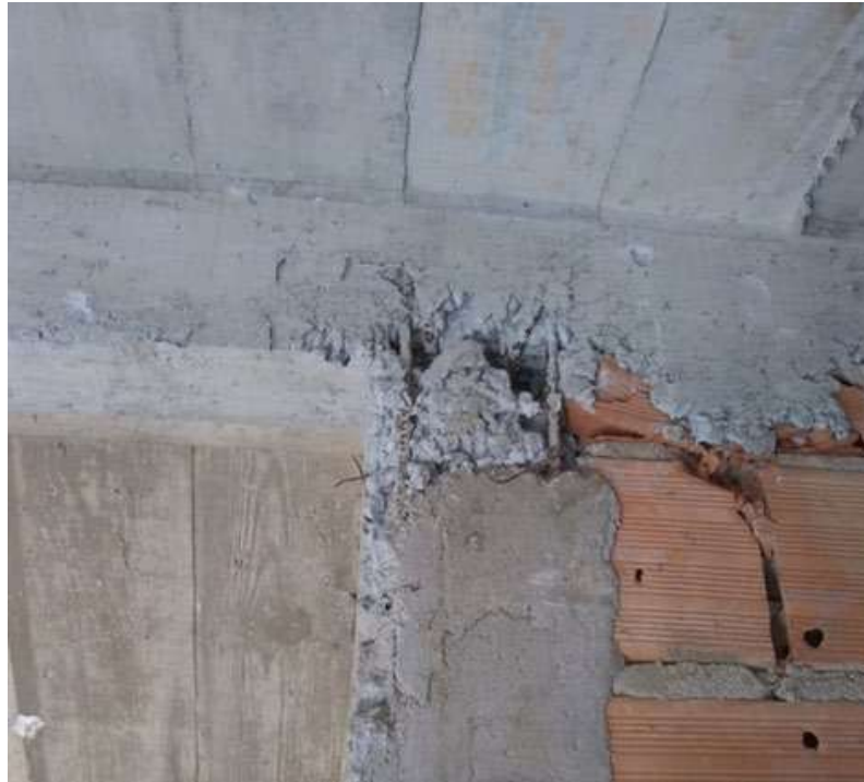
Figure 4. Drill in the beam-column connection that favors the corrosion of the reinforcement.
