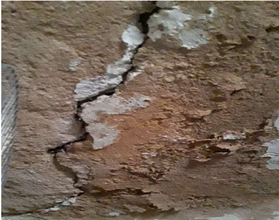
Figure 3: Crack in sealing masonry Source: Collection of authors (2021).
