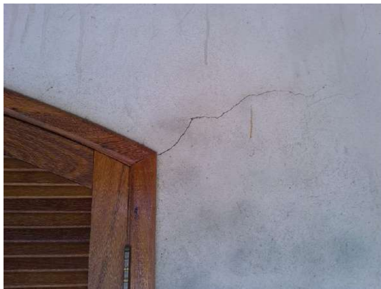
Figure 6. Crack in lintels.
