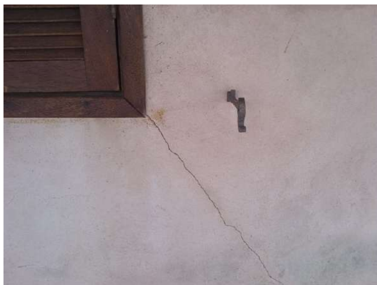
Figure 7. Crack in counter lintels.
