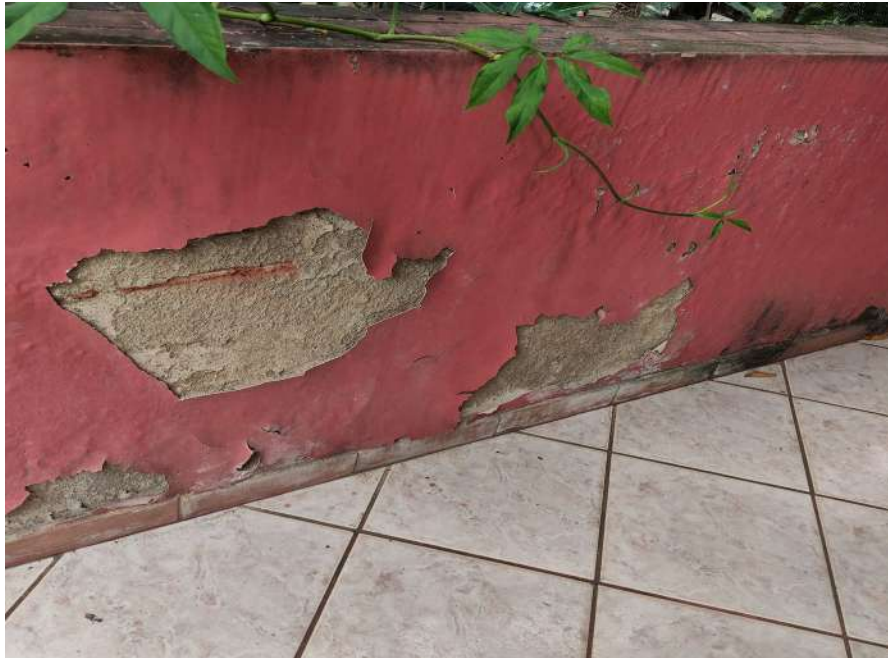
Figure 4: Coated wall showing moisture and seepage. Source: Collection of authors (2021).
