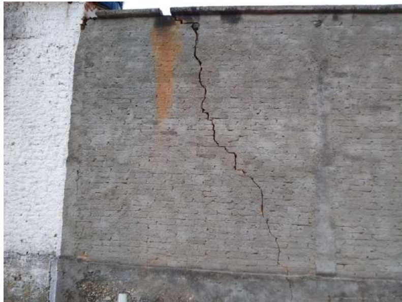
Figure 1. Crack in wall caused by settlement.
