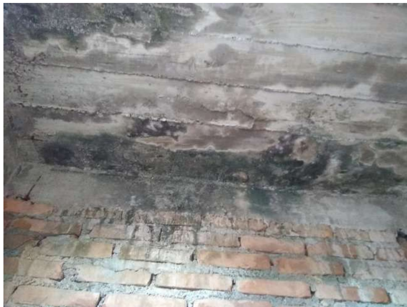
Figure 3. Reinforced concrete slab with mold and stains.
