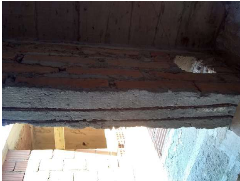
Figure 5. Exposed reinforcement in the frame support beam.
