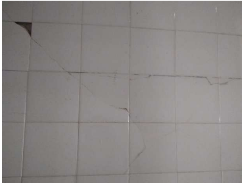
Figure 2. Cracks in ceramic tiles caused by settlement.
