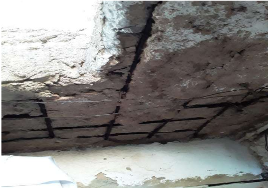
Figure 2: Structure with infiltration and corrosion of armature Source: Authors' Collection (2021).
